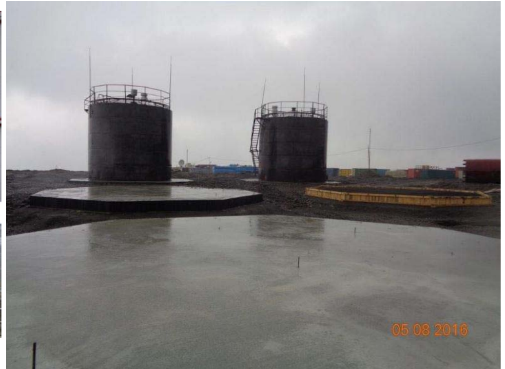
Fuel Storage Facilities – tank bases
